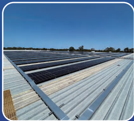
10.27 MW of rooftop solar power in the UK
