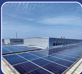
Rooftop solar power project in Accra, Ghana - 10.56 MWp
