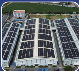
Rooftop solar power project in Khon Kaen, Thailand
